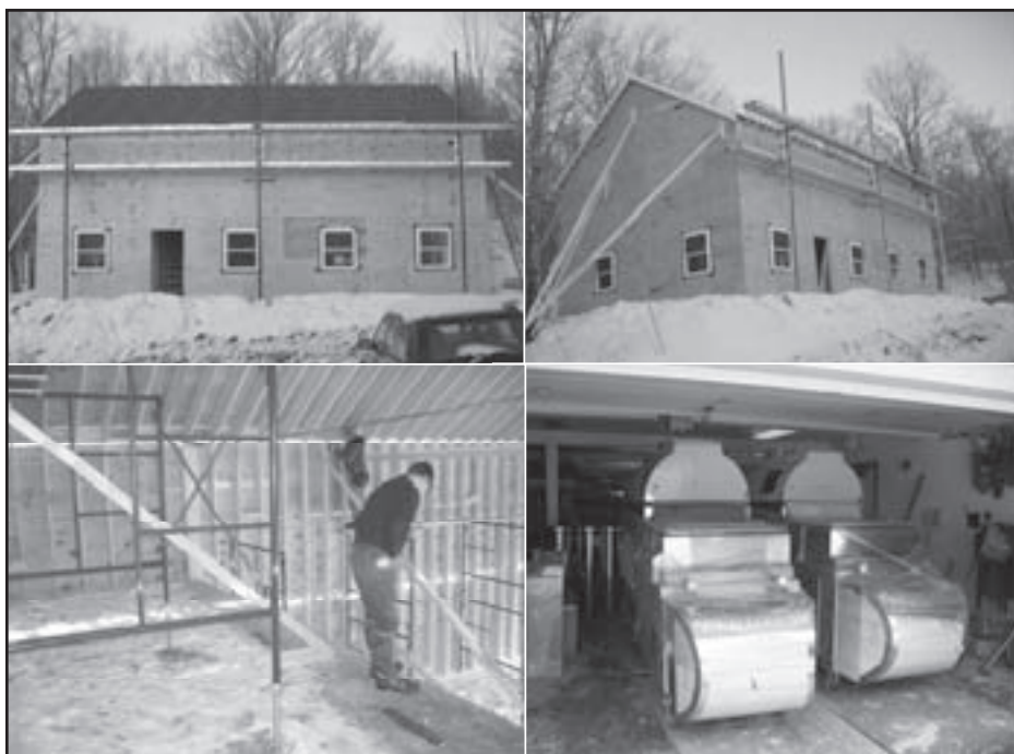
Pictured above are photos of construction progress at the new research facility located at the UVM Proctor Maple Research Center in Underhill, Vermont.
