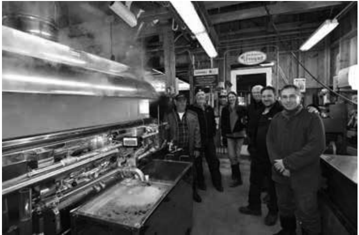
Figure 2. The Lapierre Volcano 2000 4' x 12' evaporator in the Sumner Hill Williams Sugarhouse at UVM PMRC in spring 2017. From left-right, Donald Lapierre (Lapierre Equipment), Dr. Timothy Perkins (UVM PMRC), Dr. Abby van den Berg (UVM PMRC), Jeff Goulet (Lapierre Equipment), Carl Lapierre (Lapierre Equipment), and Brian Stowe (UVM PMRC). Photo Credit: Peter Gregg, The Maple News.
