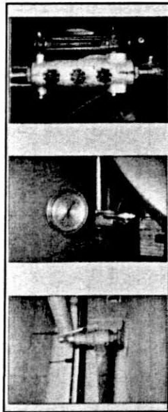
The above pictures show a Safety Relief Valve, a Steam Gauge and a Water Column in that order.
